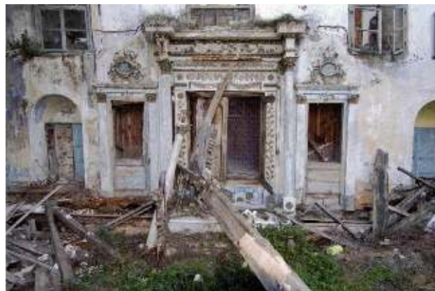
Hevra Synagogue after collapse, Internal facade, 2016
